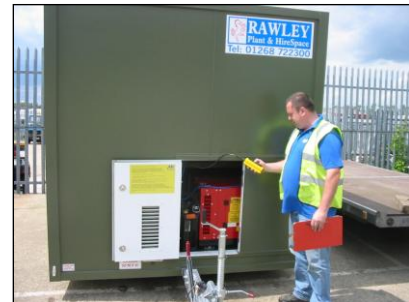
3.6m (12ft) COMBI-GEN® exterior Axel retraction in operation
